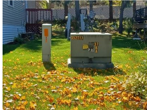
20. typical pad mounted transformer
