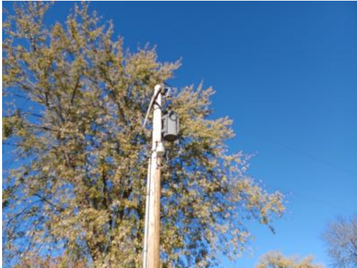
19. typical pole mounted transformer
