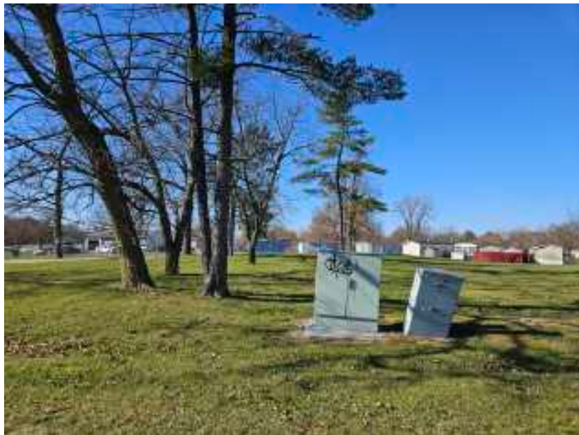
24. Pad-mounted transformer typical
