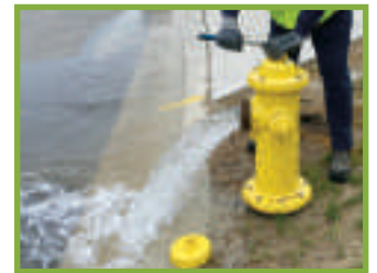
▲ In 2022, City Utilities performed maintenance on 7,943 out of 11,939 fire hydrants in Fort Wayne.
