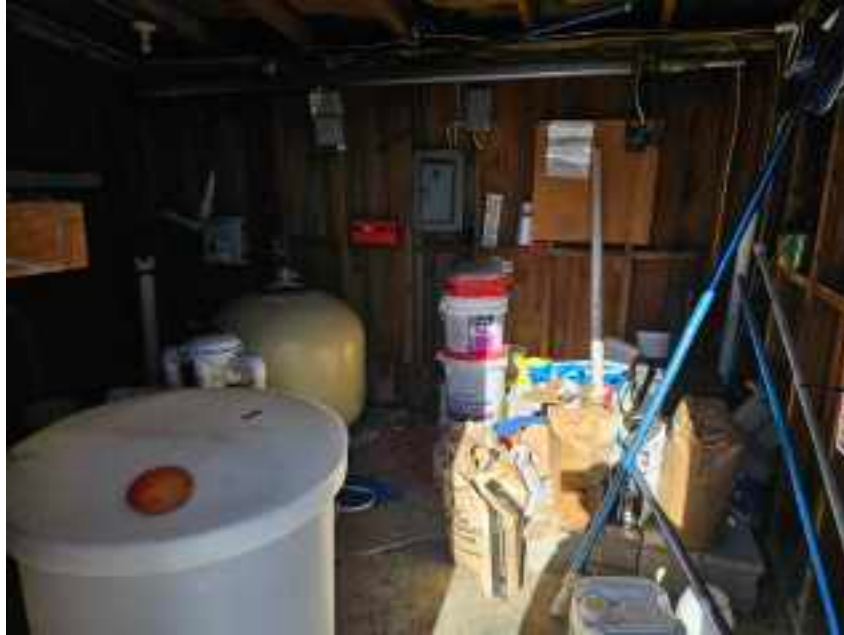
25. Pool equipment room
